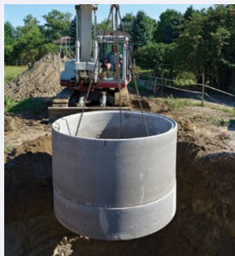
Minnetonka manages daily maintenance and capital improvement projects to provide around 300 miles each of reliable sewer and water systems.
