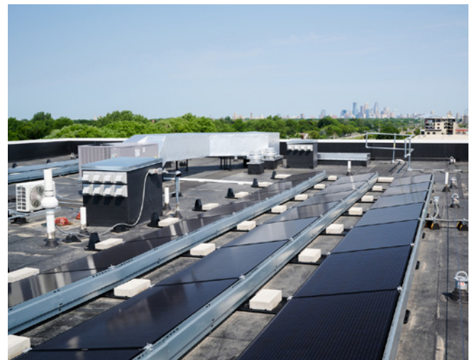
Rooftop solar – Photo by Ryan Siemers - LHB
