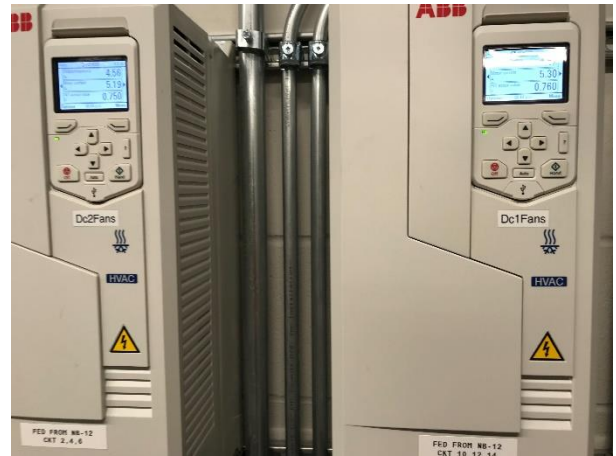
Image of cooling tower fan VFDs
