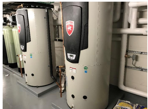
Image of service water heaters
