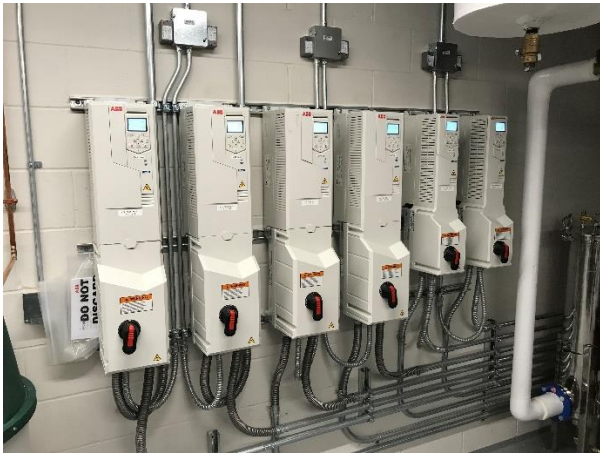
Image of typical pump VFDs
