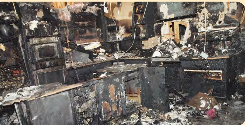
Interior damage to the Gammons' home.
