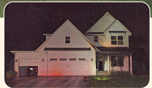
A street view reveals little damage, but the back of the home burned beyond recognition.
