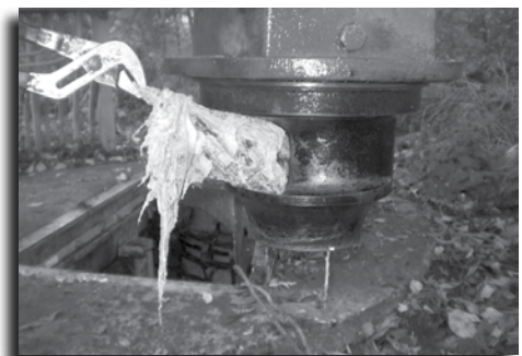
A Minnetonka sewer lift pump clogged with “flushable” wipes.
