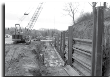
A retaining wall under construction at the Hwy. 169 and Bren Road interchange project.
