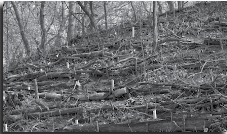
Buckthorn removal was a big part of the project. Above, buckthorn logs and branches were used to stabilize slope at the park. Photo courtesy Heather Holm.
