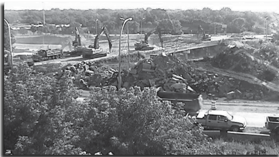
Above, demolition of Bren Road bridge. To view video of the demolition, visit www.169bren.com .
