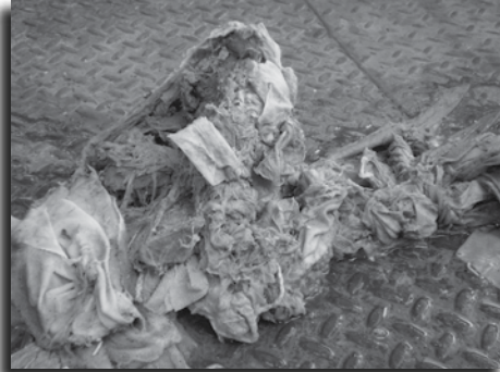
Above, a clog in a Minnetonka lift station caused by disposable and “flushable” wipes that were flushed down the toilet. These items should be placed in the trash instead.
