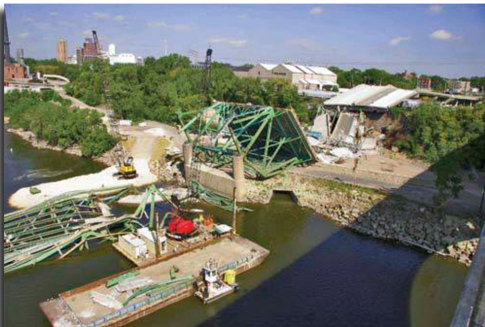
Cleanup work continues at the site of the I-35W bridge collapse in Minneapolis. Photo courtesy Jason Stenvold.
