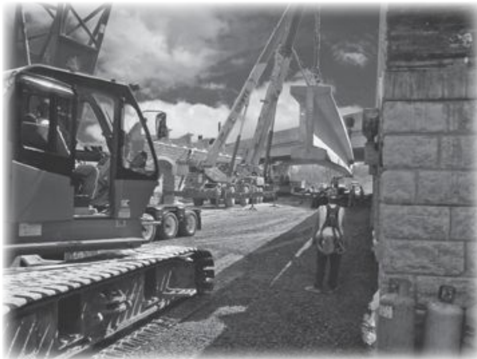
Girders for the Baker Road bridge were set last fall by MnDOT contractors.
