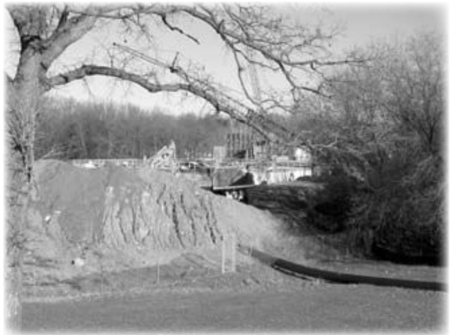
A new water treatment plant being built on the civic center campus will allow the city to provide an additional 5.5 million gallons a day of water to residents and businesses.
