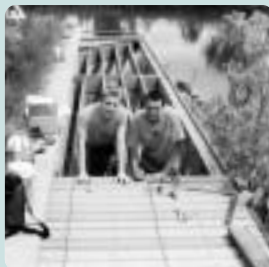
Tree Trust workers are replacing decking on the walkway adjacent to the Minnetonka Community Center.
