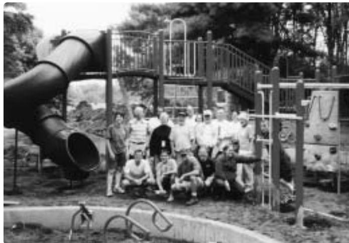
Members of Faith Presbyterian Church, neighborhood residents, and city staff joined together to install the new play equipment in Pioneer Park.
