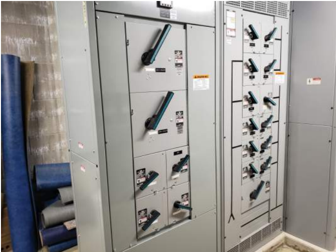
FIGURE 19: Power distribution system was observed to be in good condition.
