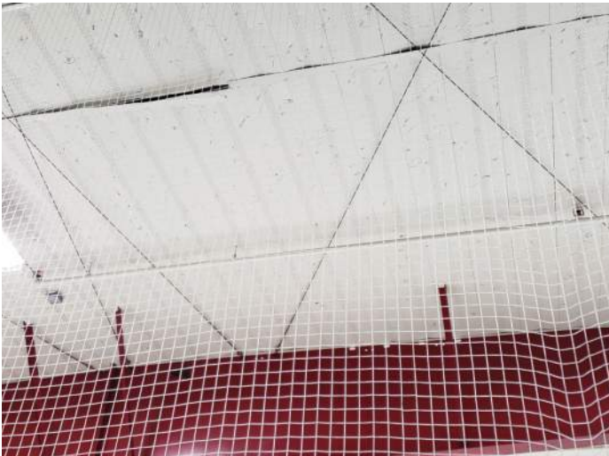
FIGURE 45: Insulation panels at underside of roof are sagging.
