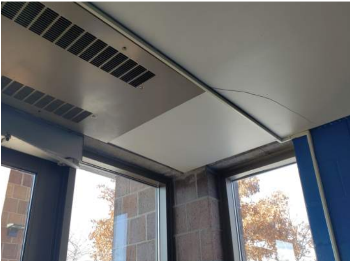
FIGURE 18: Crack in vestibule ceiling.
