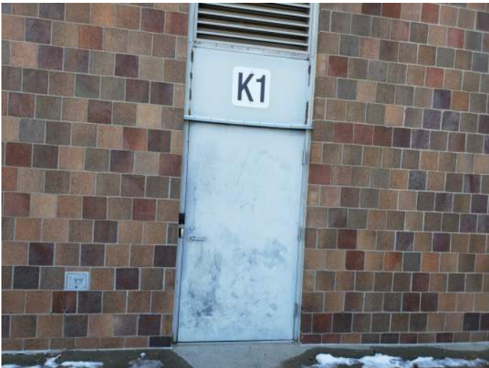
FIGURE 3: Hollow metal door and frame with poor paint finish.
