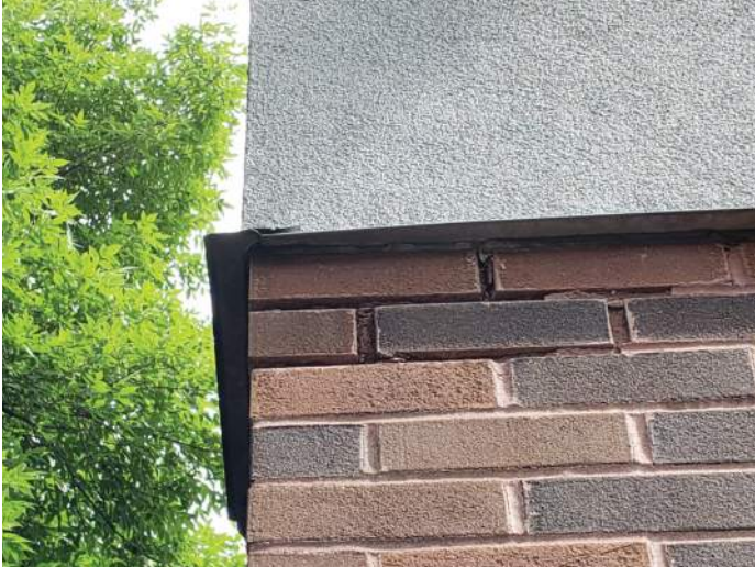
FIGURE 7: Deteriorating mortar at top of wall.
