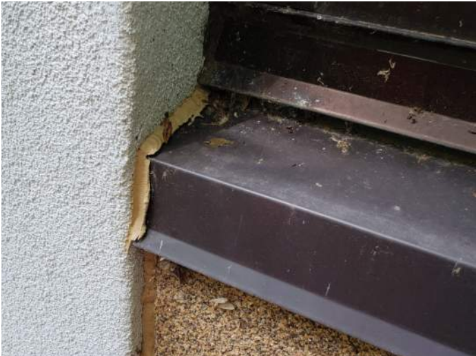
FIGURE 12: Sealants at window sills are failing and no longer adhered to the surface. Recommend replacing sealant.
