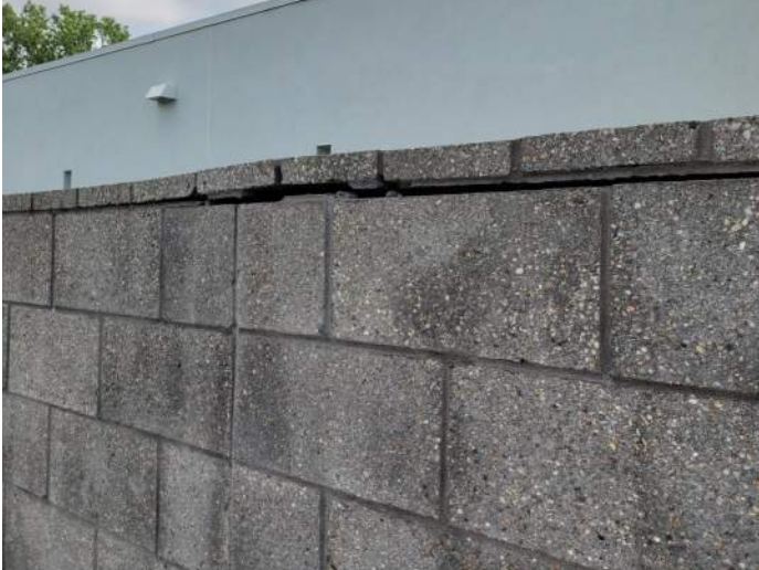
FIGURE 1: Damaged masonry cap at landscape wall adjacent to ramp. Recommend replacing cracked units and repairing cap.
