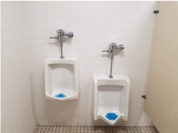
FIGURE 38: Fixture do not have automatic flush valves. Consider replacing to use less water.
