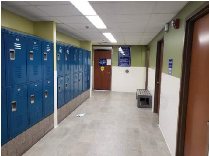
FIGURE 27: Lockers, floor, wall, and ceiling finishes are in good condition in family locker room.
