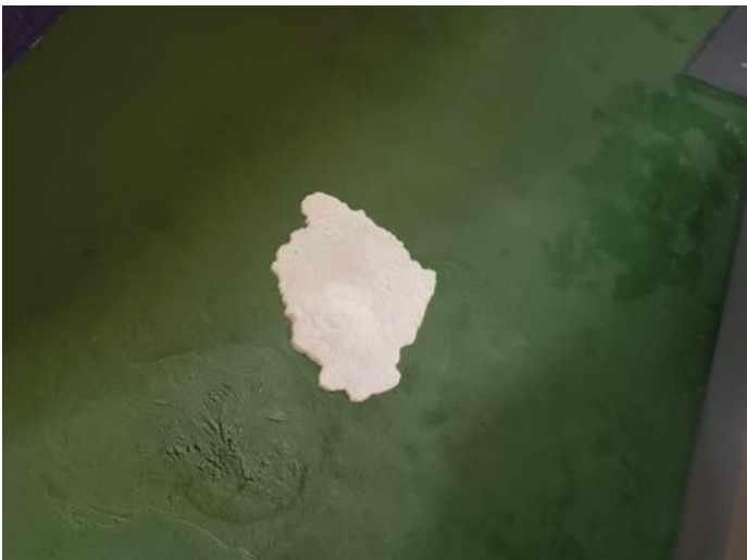
FIGURE 21: Floor finish in tennis court area is peeling.
