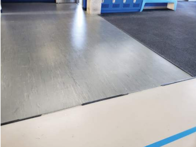
FIGURE 7: Missing/damaged floor transitions.
