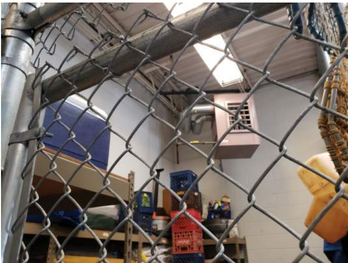
FIGURE 20: Unit heater in storage space is operational; age is assumed from 1998 remodel.
