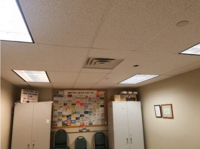
FIGURE 40: Diffusers in Oak Knoll Room were loud due to excessive amount of air coming through diffusers.
