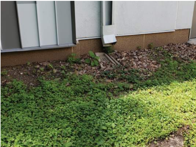
FIGURE 14: Downspout drains adjacent to base of wall. Recommend extending downspout to direct water away from building perimeter.
