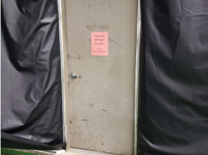
FIGURE 22: Recommend painting hollow metal door and frame and installing panic hardware for egress.
