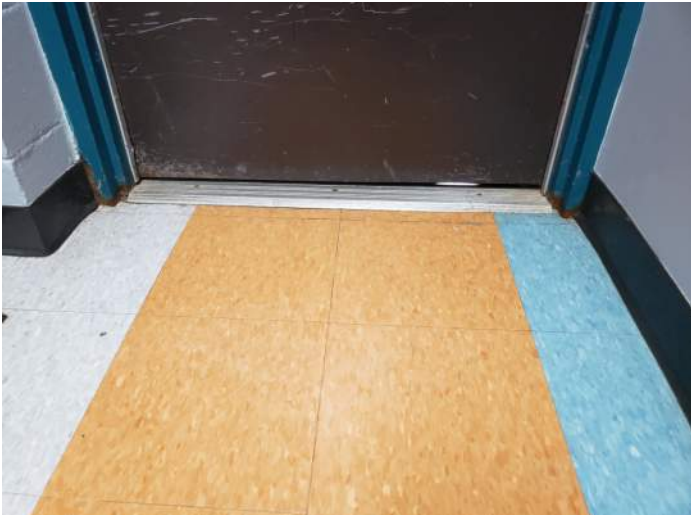
FIGURE 30: Exterior hollow metal door, damaged weather stripping and rusted. Recommend replacing weatherstripping and repainting door/frame.
