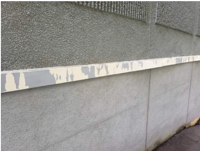
FIGURE 9: Paint at metal flashing is peeling, recommend repainting flashing.
