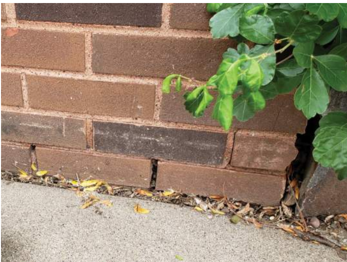
FIGURE 3: Masonry is damaged and mortar is missing at base of wall.
