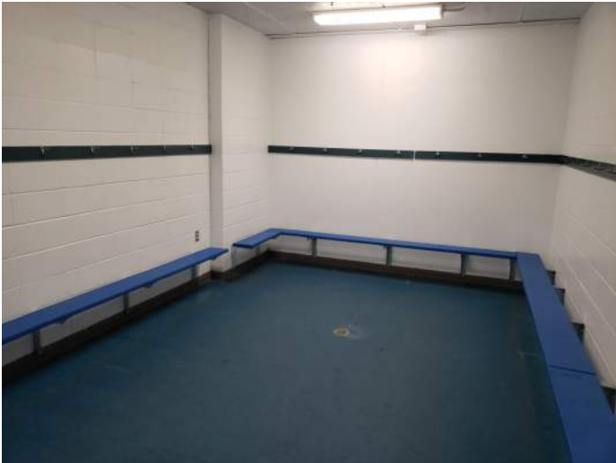
FIGURE 33: Locker room floor finishes are worn. Benches appear to be in okay condition.
