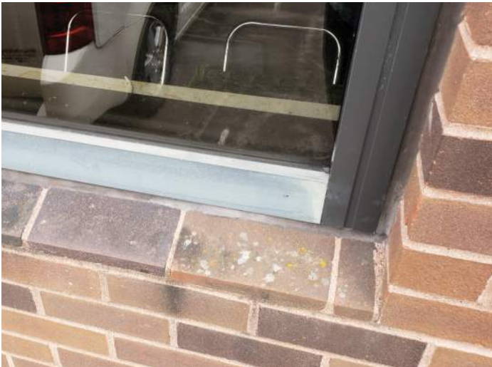
FIGURE 5: Aluminum storefront frames at punched windows are discolored, seals are dried and cracking. Recommend replacement of windows.
