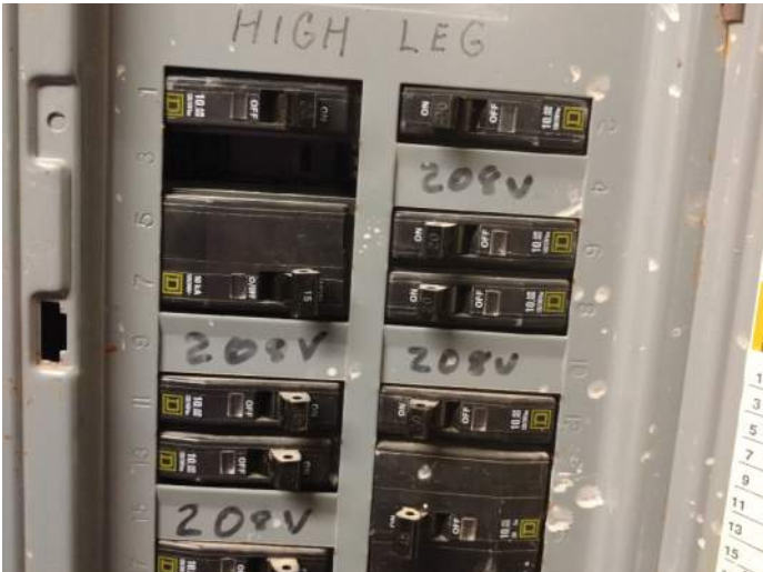
FIGURE 44: Old formerly "High Leg Delta" system panel. Now connected to 208/120V Wye system.
