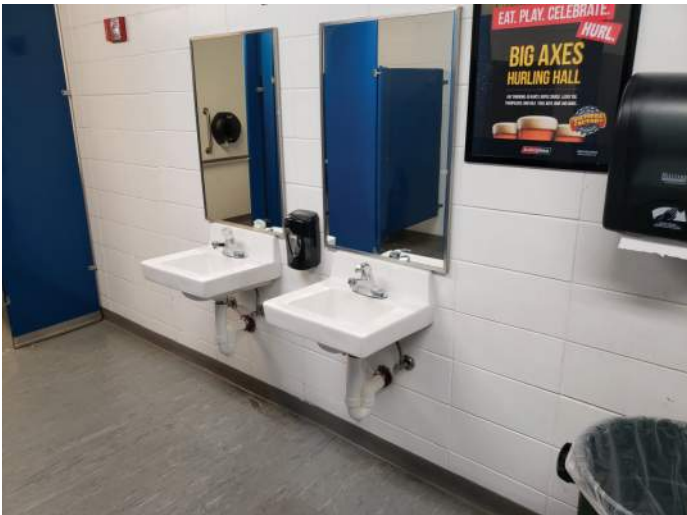
FIGURE 27: Restrooms are accessible. Finishes are worn and aged.
