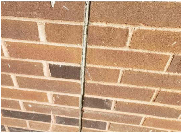
FIGURE 5: Expansion joint sealant is failing. Sealants should be replaced.
