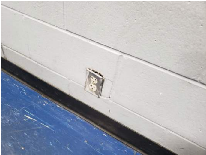
FIGURE 39: Damaged electrical receptacle, recommend replacement.
