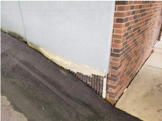
FIGURE 8: Deteriorating EIFS at base of wall.
