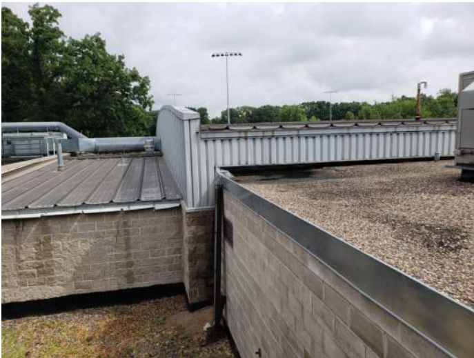
FIGURE 14: Roof has ponding water near downspout outlet. Recommend adjusting roof slope to improve drainage and install downspout extensions.
