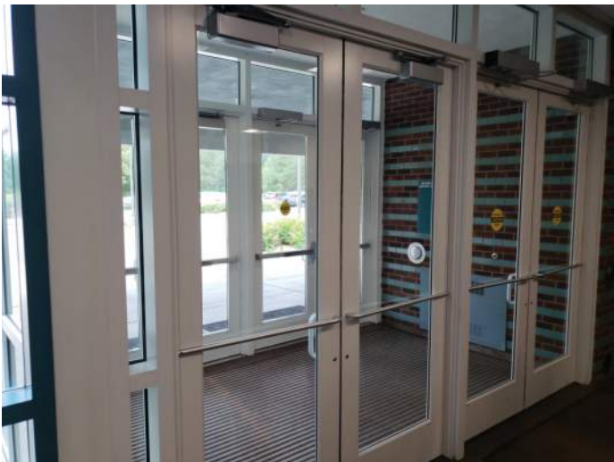
FIGURE 26: New storefront entrance installed recently, like-new condition. Doors have pneumatic powered operators installed and are in working order.
