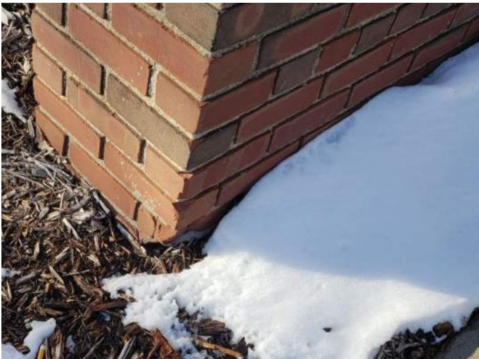
FIGURE 3: Damaged/deteriorating masonry at base of wall.
