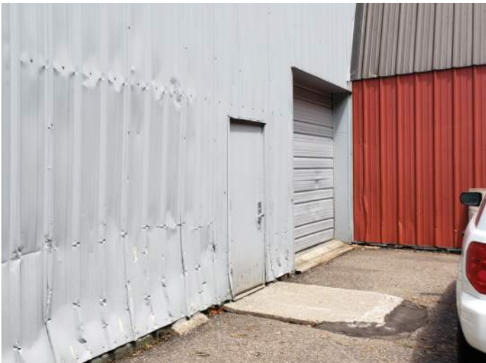
FIGURE 6: Hollow metal door is rusting. Recommend repainting door.
