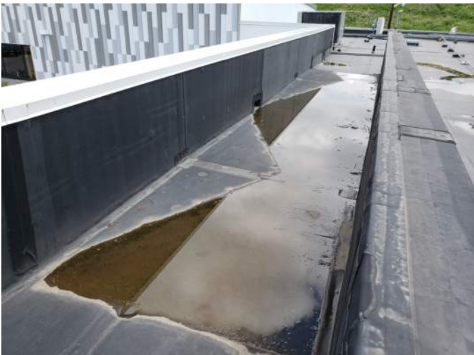
FIGURE 11: Ponding water was observed on the roof. It is recommended that water drain from roof area within 24 hours of a rain event.
