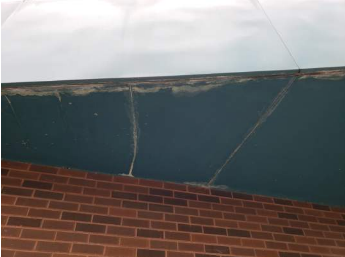
FIGURE 16: Corrosion was observed at underside of metal panels. Recommend replacement of panels to correct water intrusion issue.
