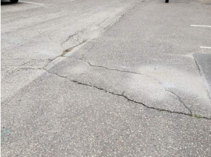
FIGURE 4: Asphalt paving is cracked and deteriorating. Asphalt paving should be patched and sealed to prolong life.
