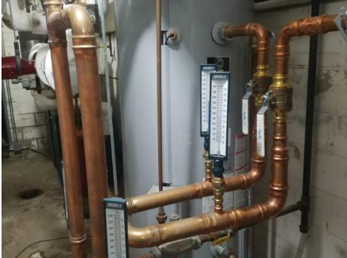
FIGURE 34: Water heaters were recently installed.
