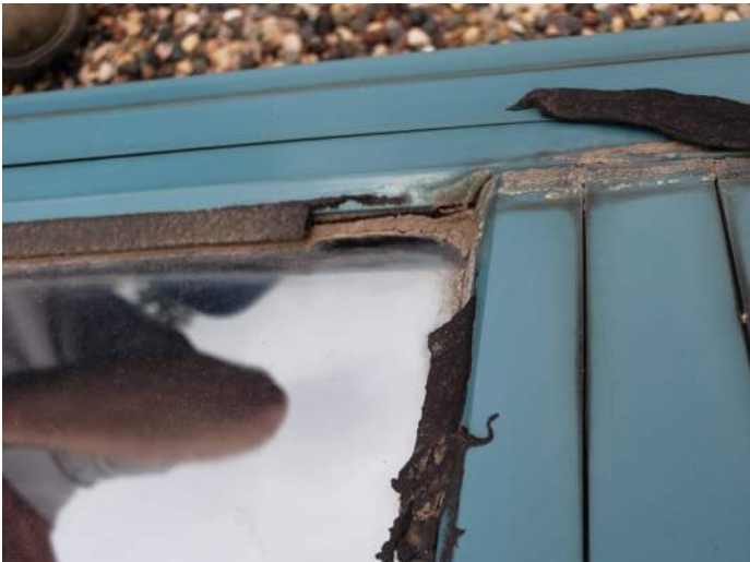
FIGURE 20: Seals at the skylights have failed, multiple attempted repairs were observed. Recommend replacing skylight glazing and seals.
