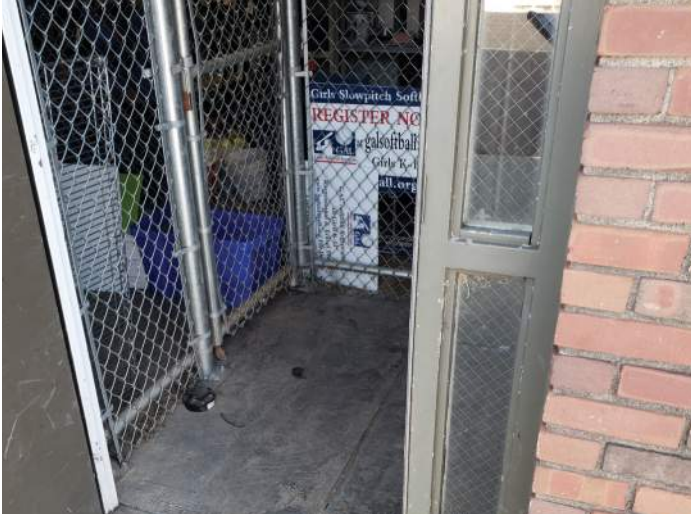
FIGURE 4: Hollow metal door and frame with faded paint finish.
