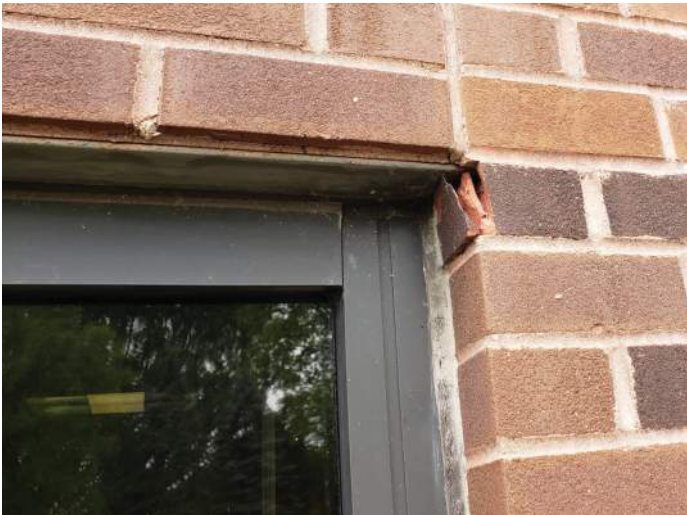
FIGURE 14: Aluminum punched windows appear to be original and are past their useful life. Damaged brick at lintel should be repaired.
