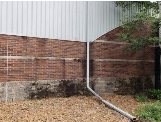
FIGURE 16: Signs of moisture on masonry wall. Recommend cleaning wall and installing drip flashing to direct water from above away from masonry below.
