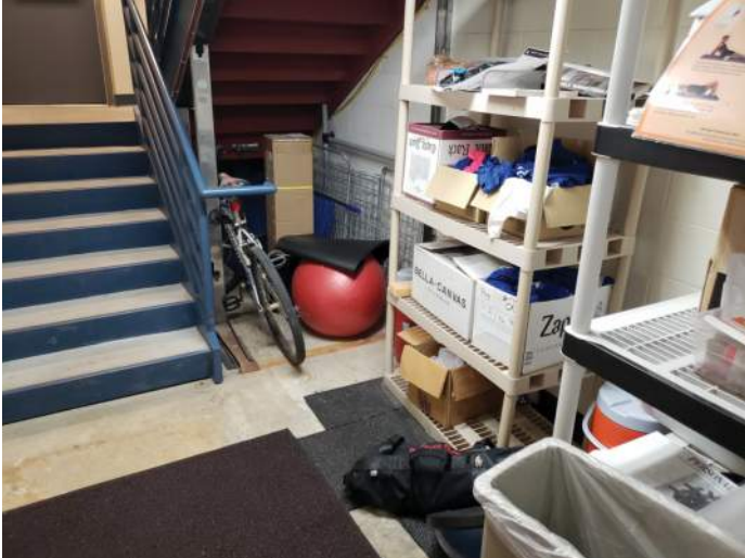
FIGURE 25: Items stored in rated stair enclosure. It is recommended that the exit stair area not be used for storage.
