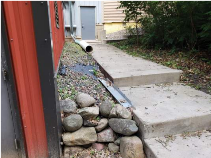
FIGURE 9: Downspout is eroding area adjacent to concrete walk. Recommend extending downspout underground to prevent further erosion.
