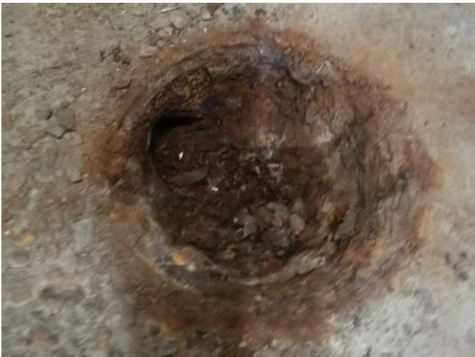
FIGURE 33: Floor drain in Boiler Room was completely corroded away.
