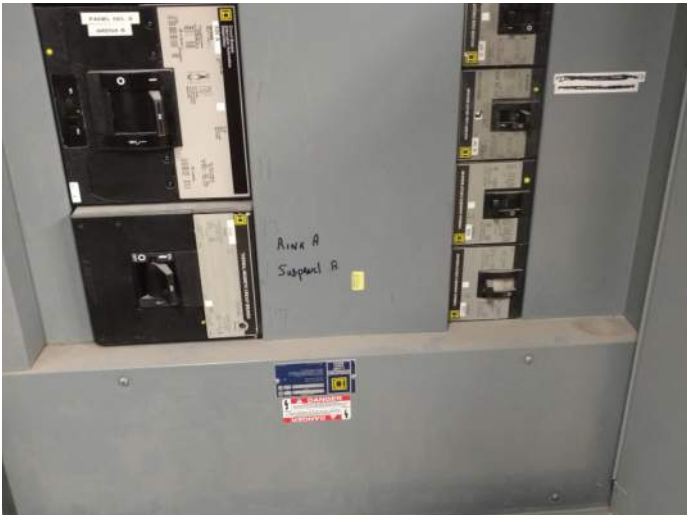
FIGURE 50: Main Switchboard and Service disconnect serving the entire building.
