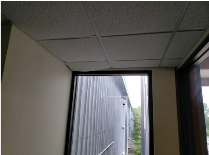
FIGURE 17: Sagging ceiling tiles in lobby.
