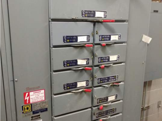
FIGURE 44: Distribution Panel for Community Center.
