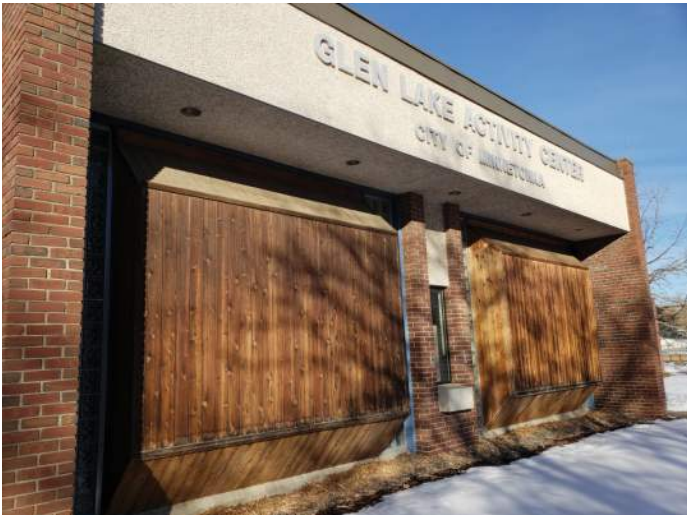
FIGURE 2: Aged/deteriorating wood siding.
