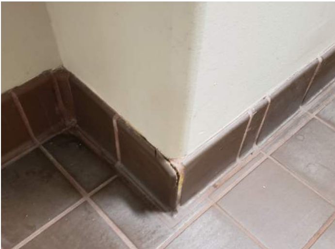
FIGURE 23: Tile floor base is cracked in lobby.
