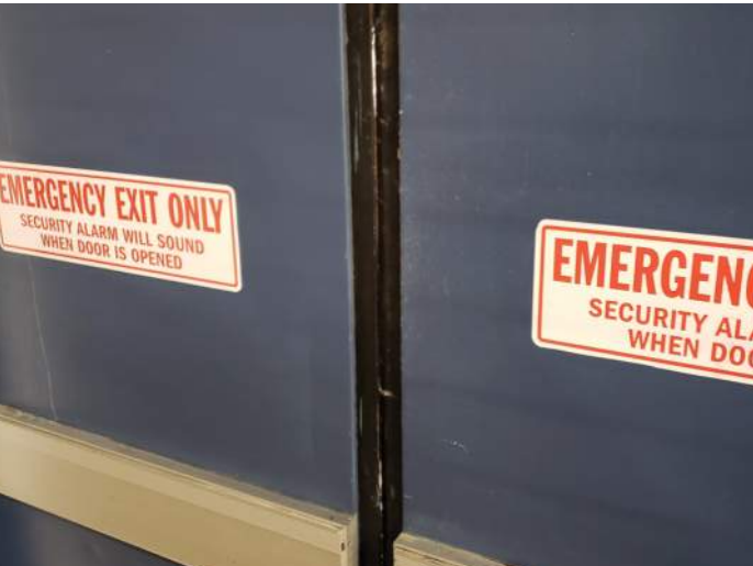
FIGURE 24: Weather seals at double door are in poor condition, light can be seen through door. Recommend installing new seals.
