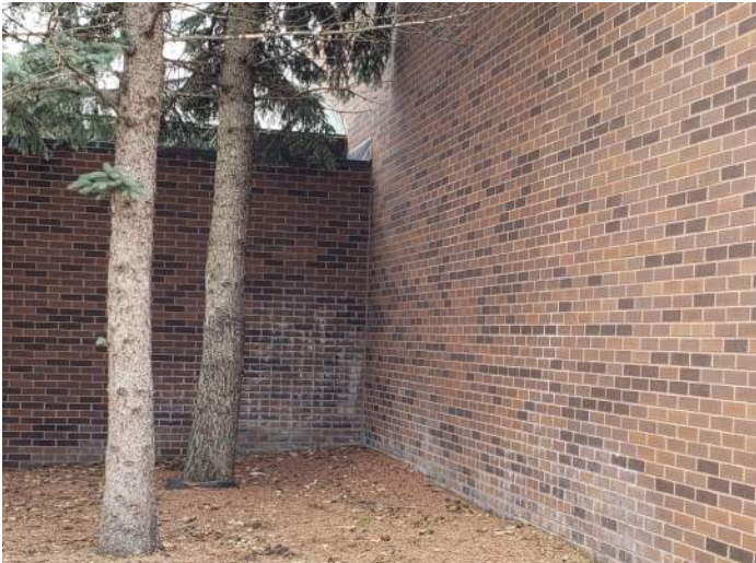
FIGURE 6: Efflorescent is visible on the masonry. Recommend adjust irrigation heads away from building and provide downspouts to direct roof stormwater.
