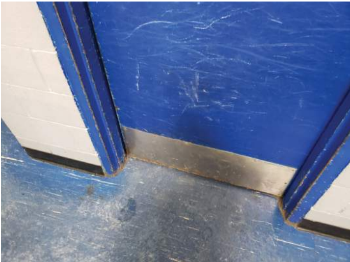
FIGURE 38: Floor finish, doors, and metal frames are in poor condition. Recommend replacing floor finish and repainting doors and frames.
