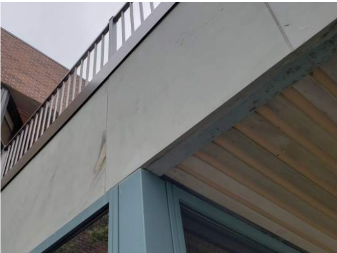
FIGURE 12: Rusted lintel at underside of deck area. Steel should be repainted to prevent further deterioration.
