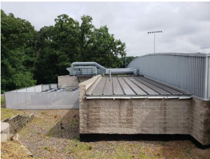
FIGURE 13: Low-slope metal roof, appears to be in okay condition. Historically roof has had numerous leaks.
