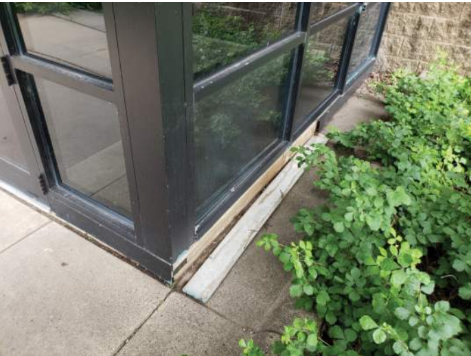
FIGURE 18: Metal sill trim piece is not attached, wood is exposed. Recommend repair to conceal exposed wood.
