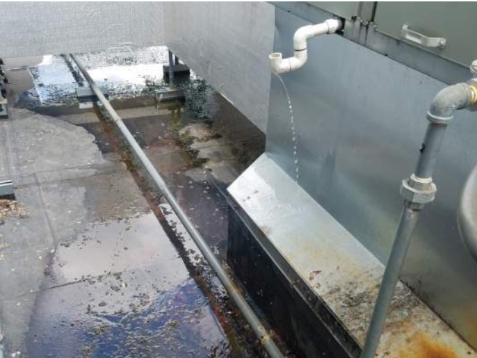
FIGURE 42: Consider having condensate picked up by drain or pump instead of flowing onto equipment and roof. This will reduce the build up on unit and roof.
