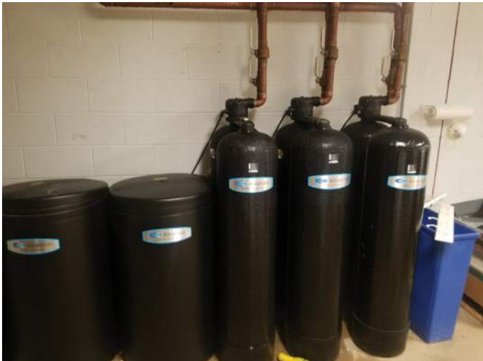
FIGURE 35: Water Softeners were recently installed.
