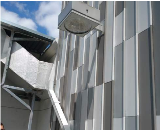
FIGURE 45: Large metal halide exterior wall-pack fixture.
