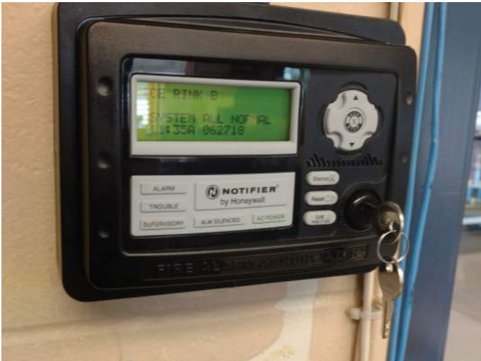
FIGURE 51: New Notifier Fire Alarm Annunciator Panel.
