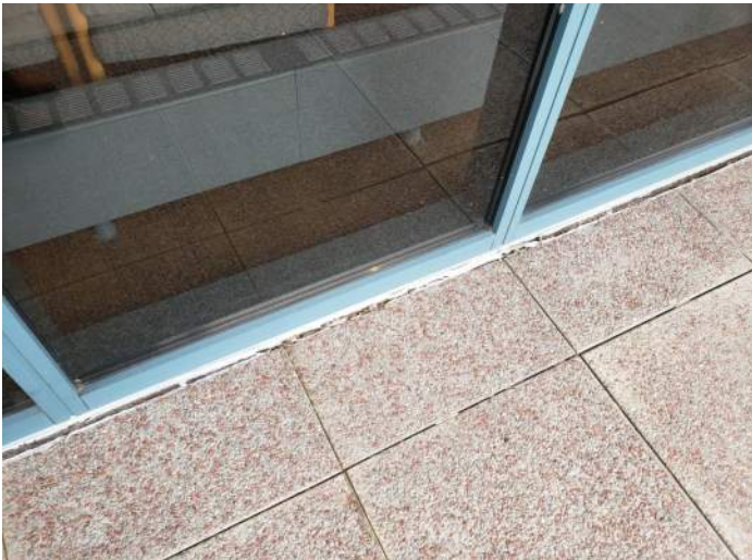
FIGURE 18: Sealant along base of wall has failed and should be replaced.
