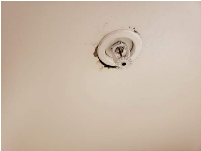
FIGURE 26: Signs of rust and moisture around ceiling mounted sprinkler head.
