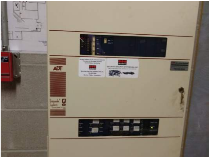
FIGURE 43: ADT Fire Alarm Panel
