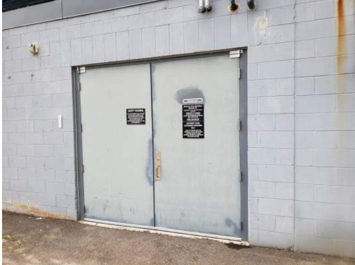
FIGURE 10: Paint on hollow metal doors and frames is faded, recommend repainting.
