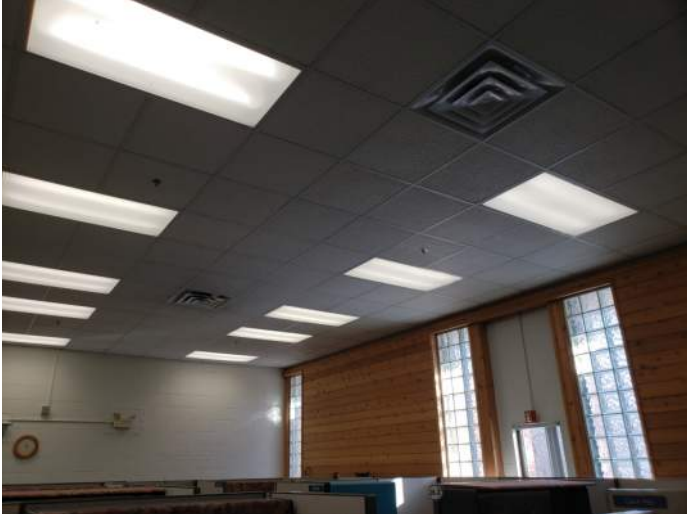
FIGURE 7: LED lamps in meeting room.
