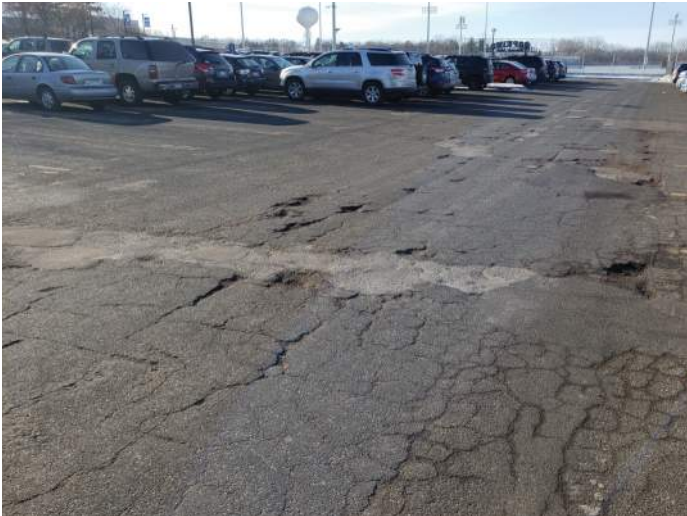
FIGURE 1: Cracks and pot holes in parking lot.
