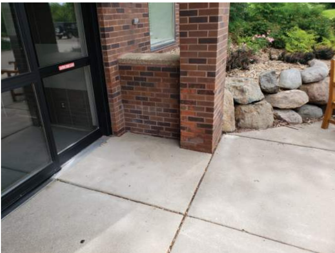
FIGURE 2: Masonry is spalled and show signs efflorescence at entry to Arena A.
