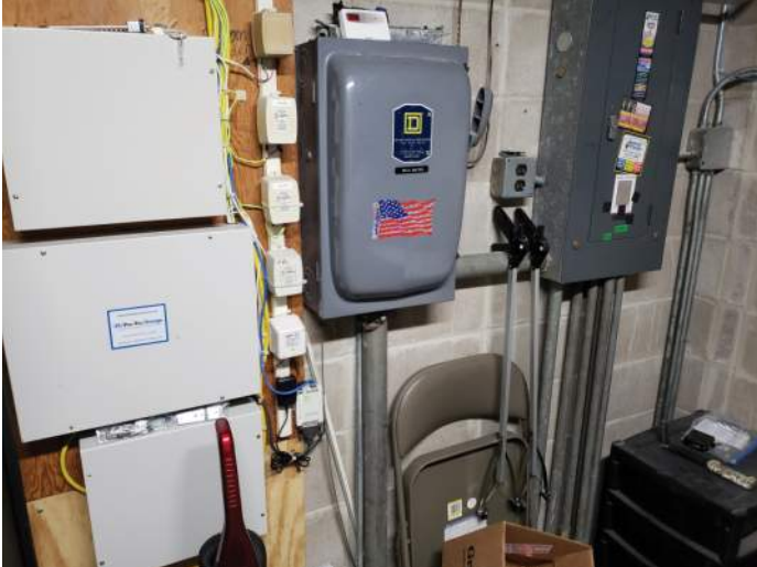
FIGURE 13: 200A electrical service.
