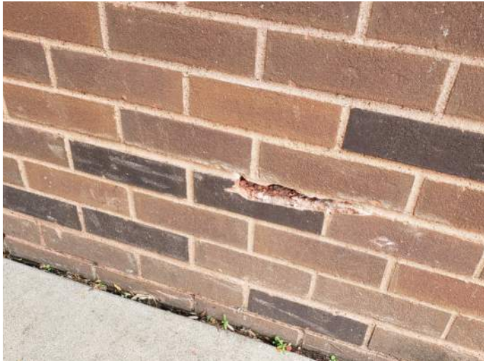
FIGURE 4: Brick is deteriorated.
