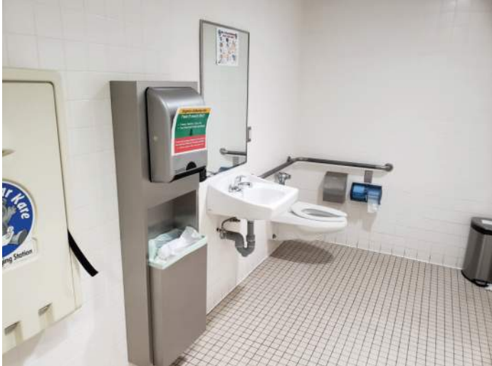
FIGURE 34: Accessible family restroom. Vertical grab bar is missing at water-closet, recommend installing grab bar to comply with MN Accessibility Code.
