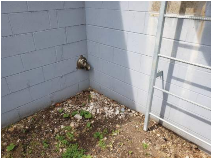
FIGURE 11: Drain empties adjacent to building, recommend extending drain to direct water away from building perimeter.
