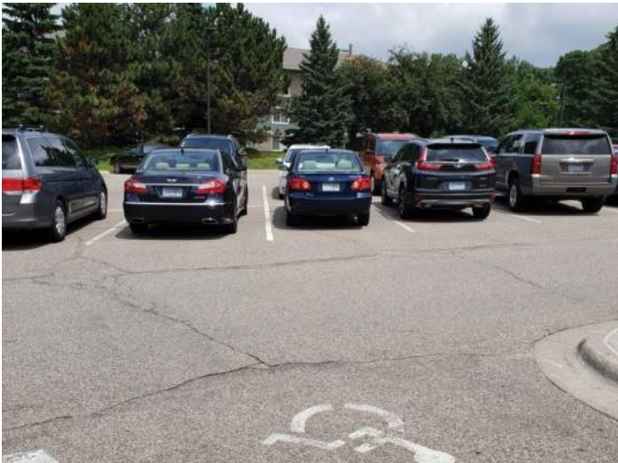
FIGURE 15: Asphalt parking area is cracking. Recommend patching and sealing parking area to extend life.
