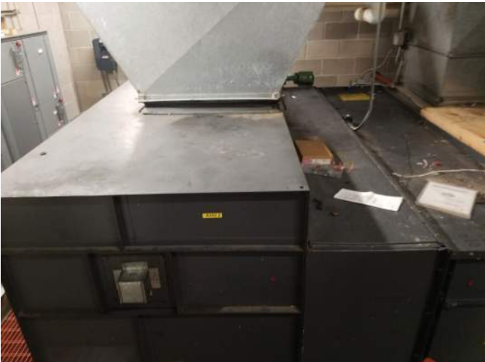
FIGURE 41: Both AHUs are past useful life, consider replacing.
