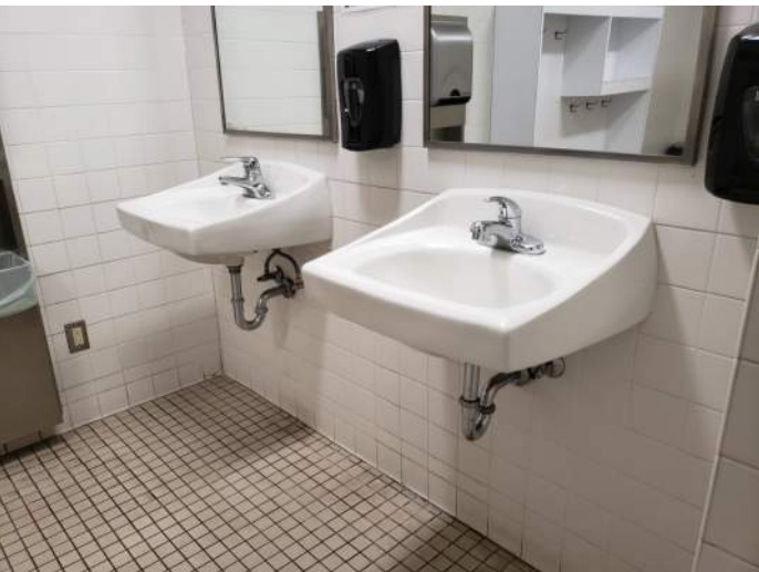
FIGURE 29: Public restrooms are not fully accessible. Lavatories require pipe protection.
