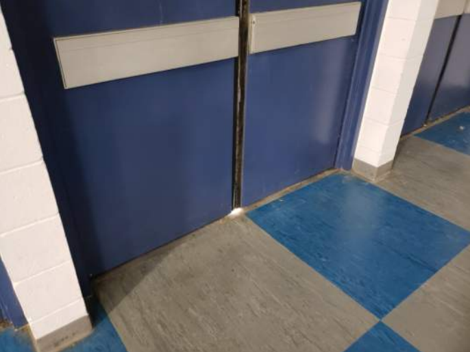
FIGURE 28: Weather seals missing at doors. Recommend installing new seals.
