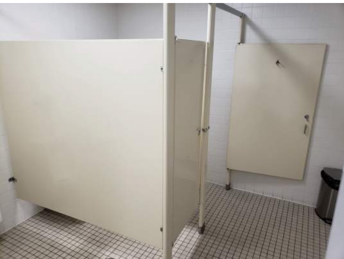
FIGURE 30: Public restrooms are not fully accessible. Waterclosets do not provide required clearances.
