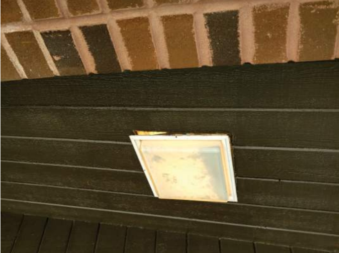
FIGURE 52: Exterior incandescent fixture. Fixture is filled with bugs and cover/lens is beginning to come apart.
