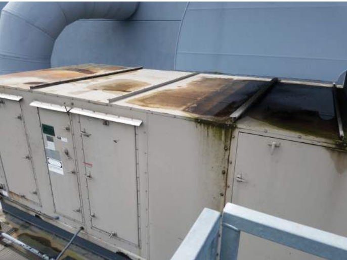
FIGURE 47: Condensate build up on AHU do to exhaust air blowing directly at unit. Consider directing air in different direction.
