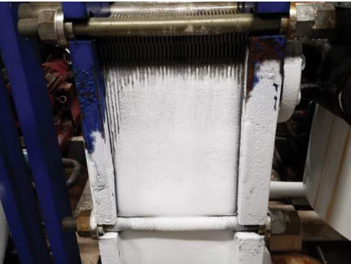
FIGURE 48: Heat exchanger for ice system in Arena B is iced up, this reduces efficiency and can cause maintenance issues.
