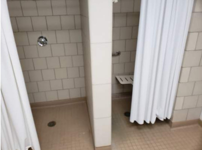
FIGURE 16: Locker room showers - finishes observed were in good condition. One shower is equipped for ADA.
