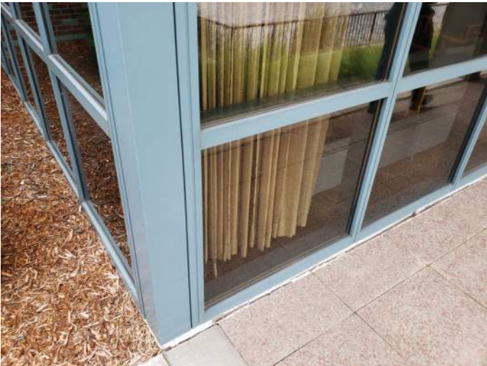
FIGURE 11: Seals at storefronts are dried and cracked. Fogged glazing was observed at several locations. Recommend replacement of seals & glazing.
