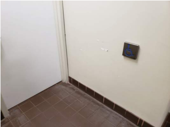
FIGURE 25: Walls are damaged in a few locations. Recommend installing chair rail or durable wainscot along walls in high traffic areas.
