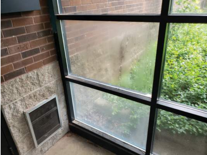
FIGURE 19: Several window panels show signs of moisture between the glass panes. Recommend replacing glazing.
