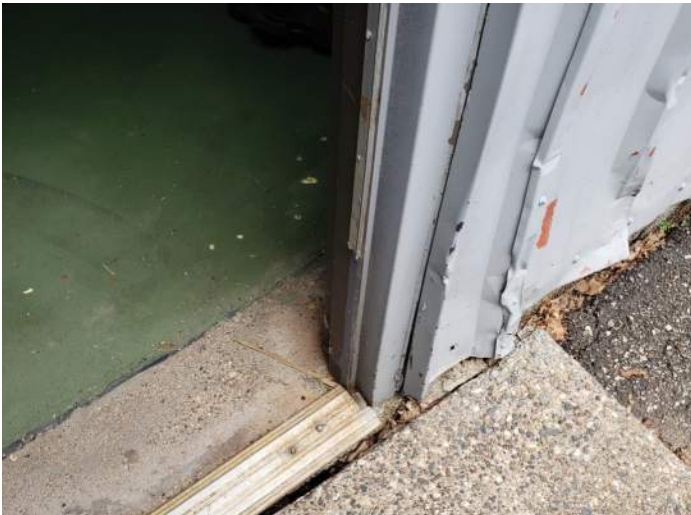
FIGURE 23: Damaged/missing weather stripping at exterior door. Recommend replacing weather stripping and painting door and frame.
