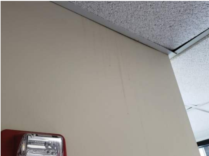
FIGURE 18: Water stains at top of wall in lobby area.
