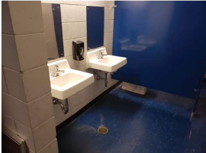
FIGURE 42: Women's restroom does not comply with MN Accessibility Code requirements. Finishes are worn.
