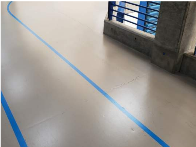
FIGURE 21: Walking/jogging track surface is cracking and peeling.
