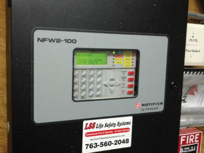
FIGURE 46: Notifier Fire Alarm System.
