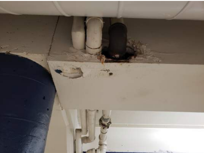
FIGURE 29: Corrosion at pipe chase in lobby. Recommend verifying pipe is not leaking and repair finish around pipe.
