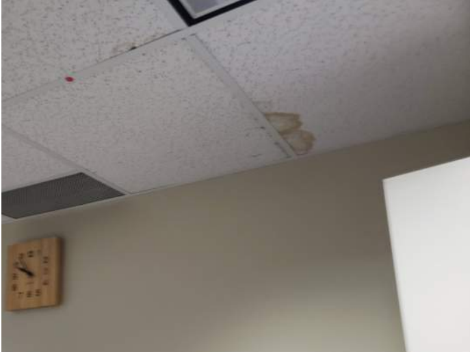
FIGURE 31: Old, stained ceiling tiles in Burwell Room and staff areas. Leak is believed to already been corrected. Recommend replacing ceiling tiles.
