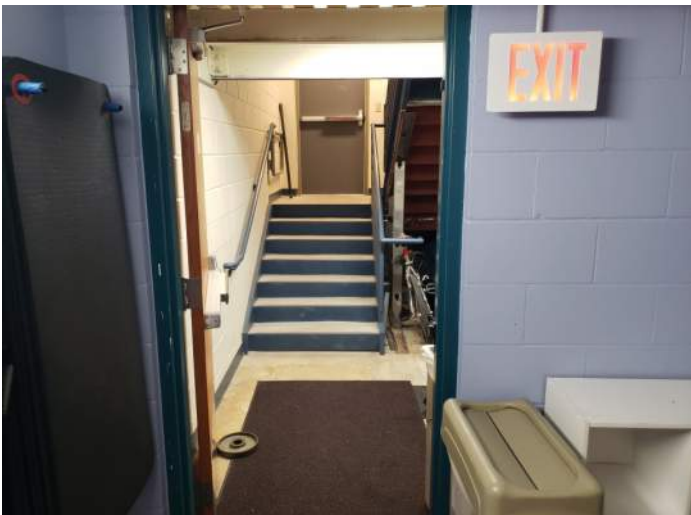
FIGURE 24: Fire-rated exit door held open. Door is part of rated enclosure and should be closed at all times.
