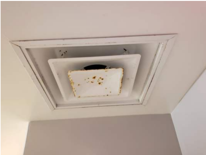
FIGURE 32: Diffuser in locker rooms is rusted. Recommend reviewing dehumidification system to improve air quality in space.
