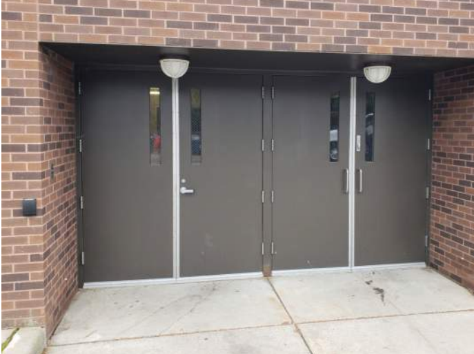
FIGURE 1: Hollow metal doors and frames are showing signs of rust and should be repainted.
