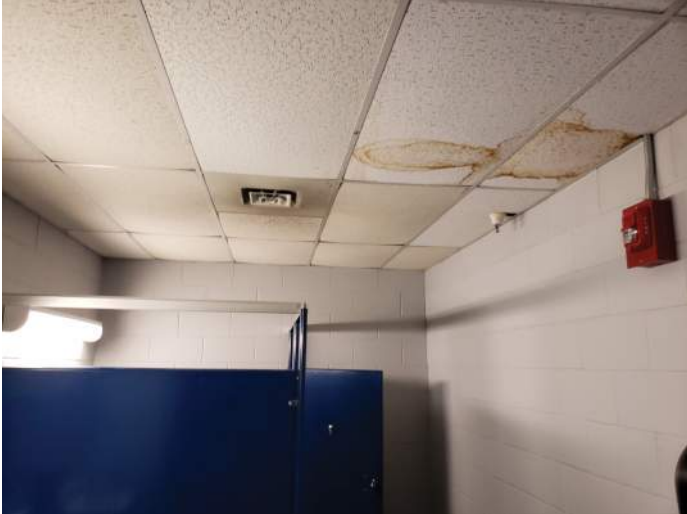
FIGURE 43: Stained ceiling tiles in Women's restroom. Recommend verifying if leak exists and repair. Replace ceiling tiles for improved appearance.
