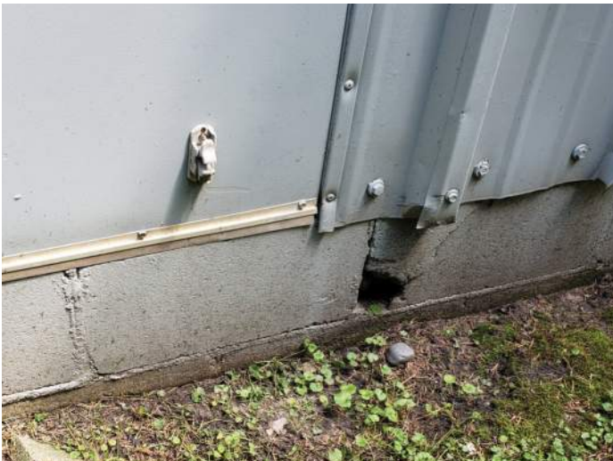
FIGURE 3: Hole in CMU masonry at base of wall. Recommend patching hole.
