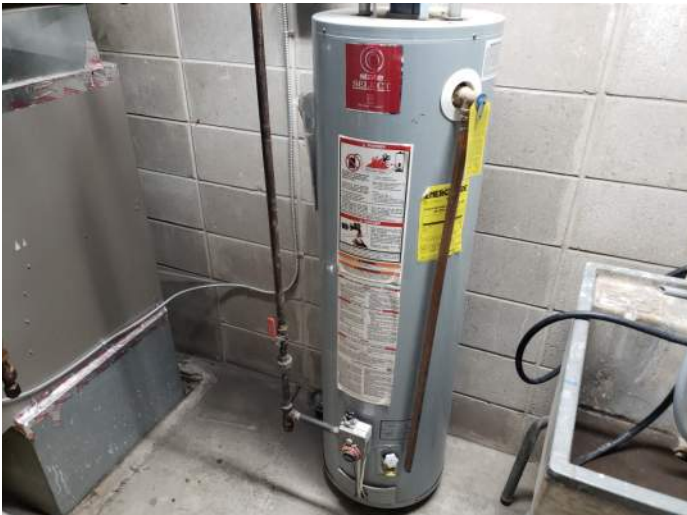
FIGURE 14: Existing gas water-heater; water-heater is past its expected life-span.
