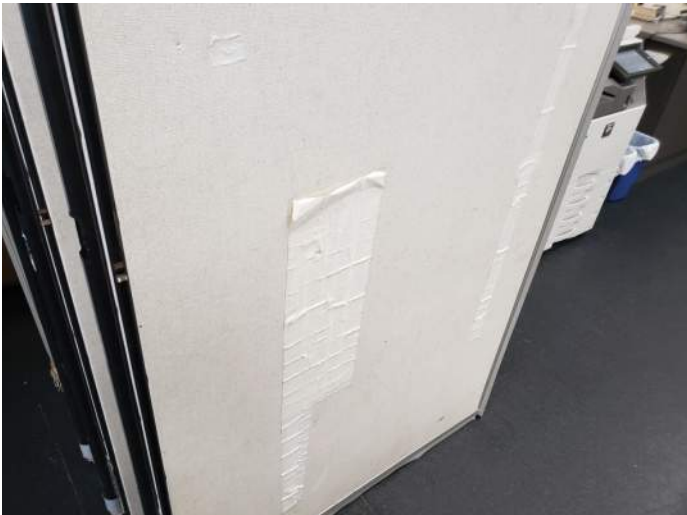
FIGURE 8: Damaged operable wall partition.
