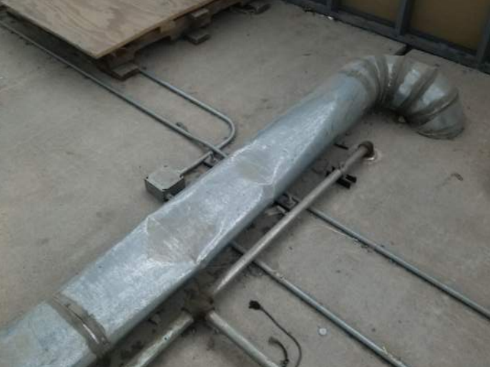
FIGURE 46: Ductwork is smashed in areas. Reform duct to proper shape.
