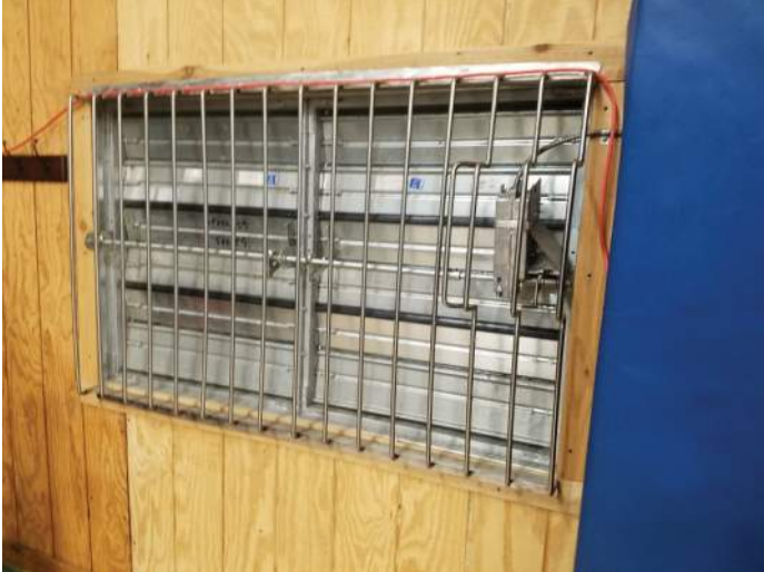
FIGURE 38: Relief dampers are all manual, consider changing these to automatic to work with exhaust fans.
