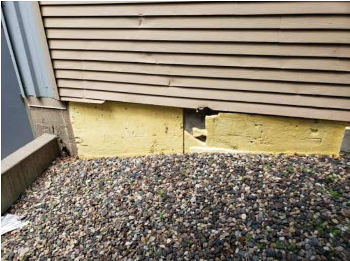
FIGURE 10: Damaged vinyl siding and deteriorating rigid insulation. Recommend replacing insulation and covering the panels with a protective material.
