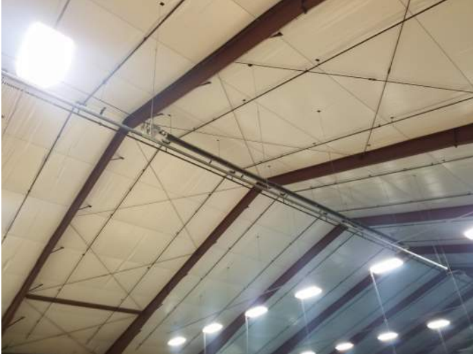
FIGURE 37: Tennis court is served by a single radiant heater. Consider installing multiple, along with destratification fans.
