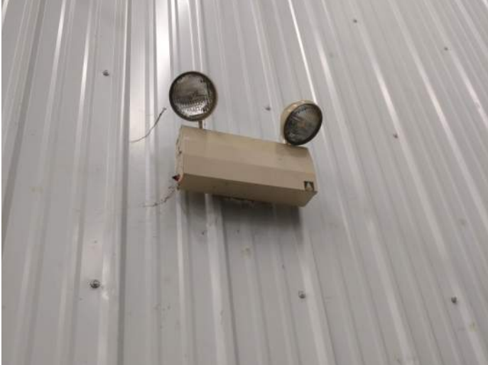
FIGURE 43: Old remote head emergency light fixture.
