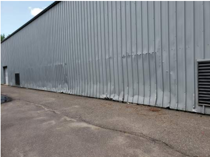
FIGURE 5: Metal wall panels are damaged at backside of building.
