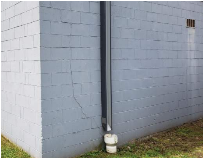
FIGURE 12: Crack in masonry wall, recommend patching crack.
