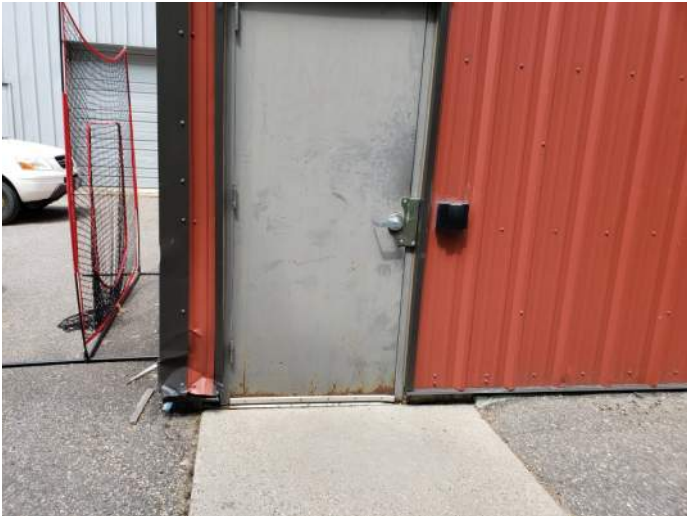
FIGURE 7: Hollow metal door is rusting and metal panel is damaged at outside corner. Recommend installing a bollard to protect building and repaint door.
