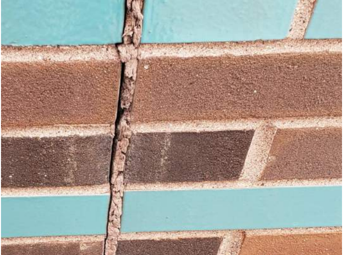
FIGURE 7: Deteriorated expansion joint sealant at masonry wall. Sealant at expansion joints should be replaced to avoid water from entering wall.
