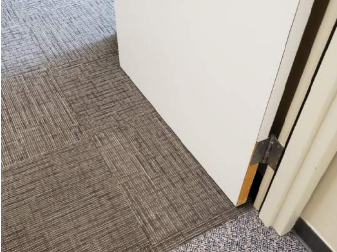
FIGURE 32: Old carpet finish and delaminating doors in staff areas. Recommend replacing doors and carpet finish.
