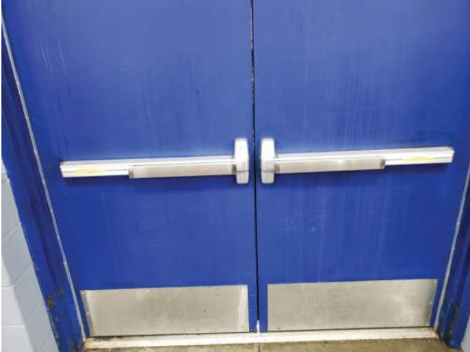
FIGURE 37: Exterior doors lacking weather seals, recommend installing new weather seals.
