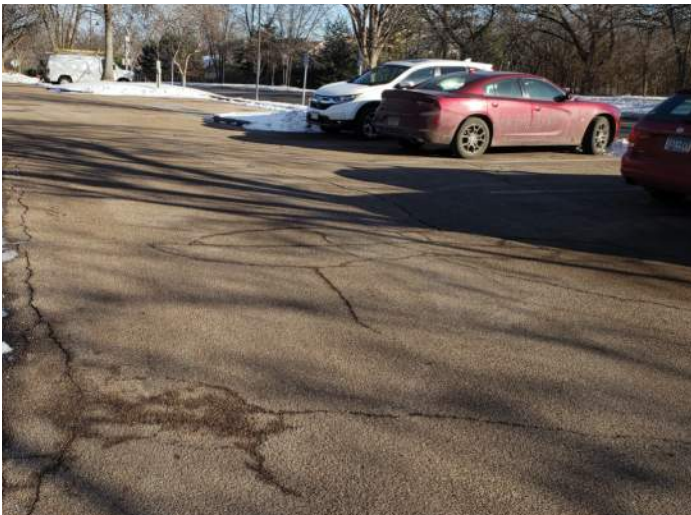
FIGURE 6: Cracks in asphalt parking area.
