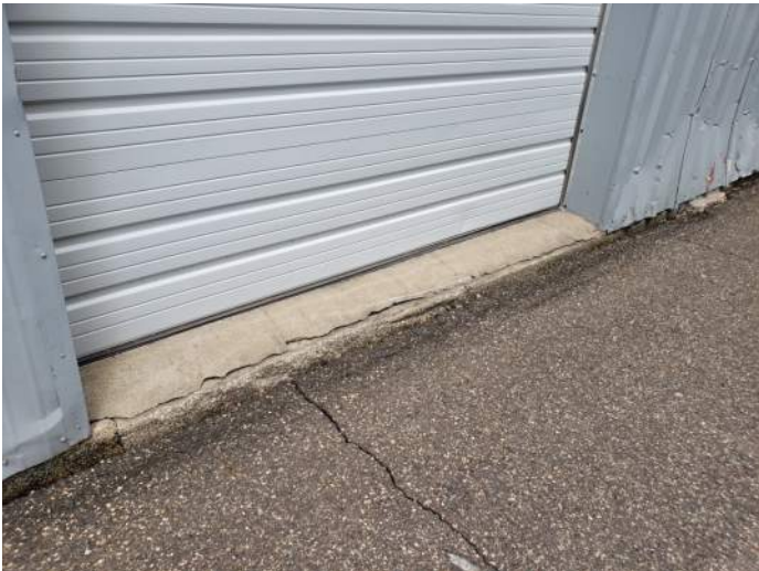
FIGURE 2: Cracked and chipped concrete stoop at overhead door. Cracked asphalt paving.
