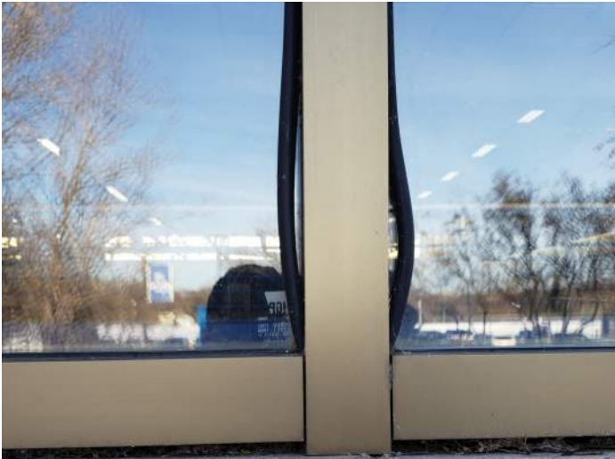
FIGURE 4: Glazing seals at aluminum storefront failing.
