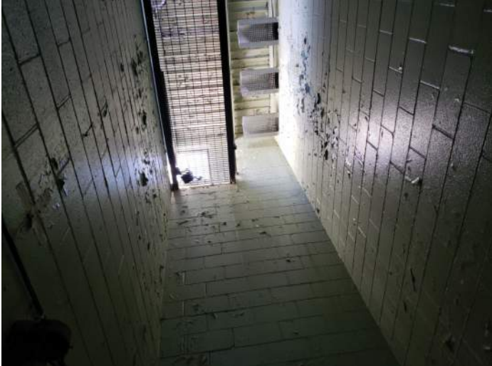
FIGURE 10: Peeling paint within hose tower.
