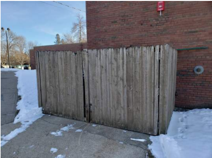
FIGURE 5: Damaged and deteriorating wood fence at trash enclosure.
