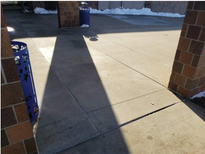
FIGURE 2: Uneven and cracked concrete at entrance.
