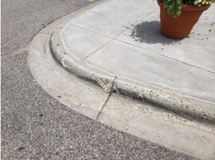
FIGURE 16: Chipped concrete curb and gutter at parking lot.
