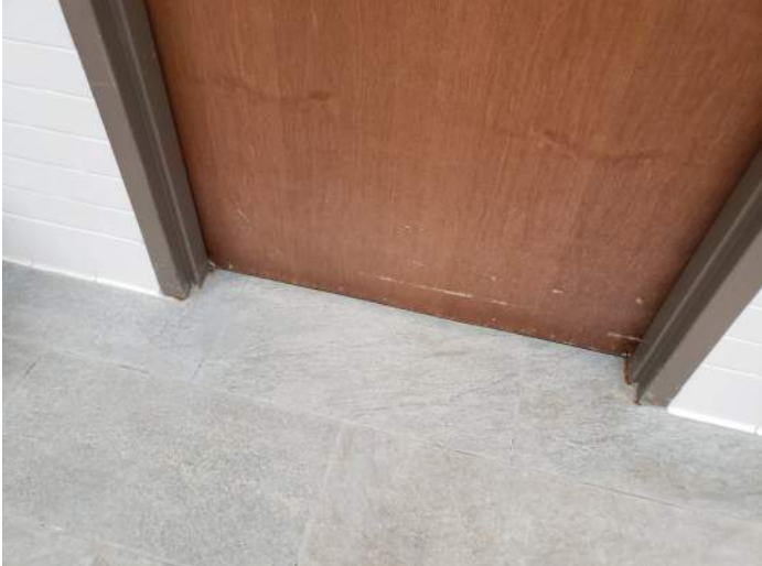
FIGURE 28: Wood doors in locker room are showing signs of moisture damage at bottom. Hollow metal frames should be repainted where rusting.
