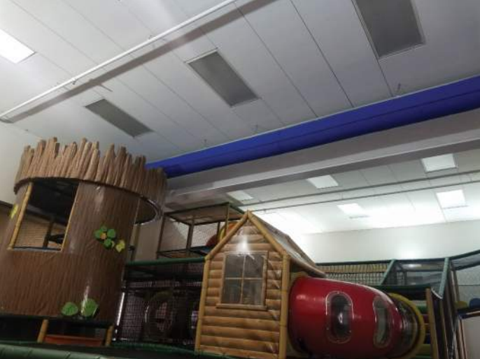
FIGURE 40: Soft duct is difficult to clean. Consider replacing with hard duct for easier access.
