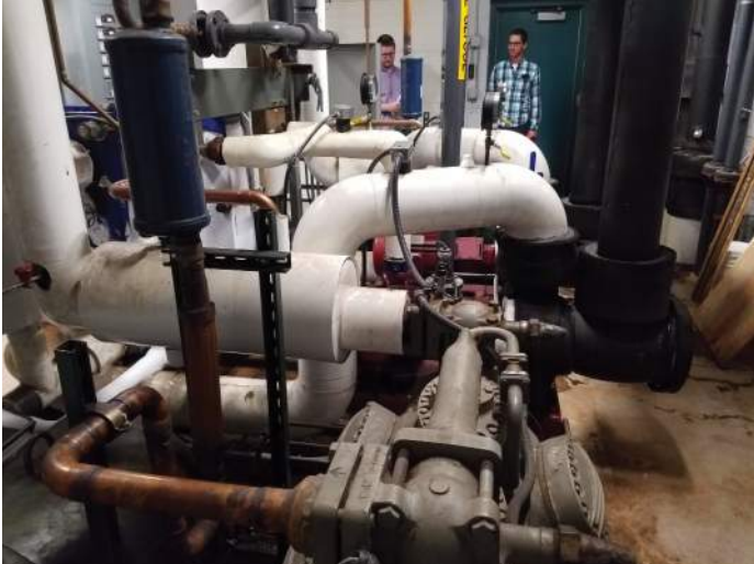
FIGURE 49: Arena B ice system is 15-20 years old and contains R-22, which will be phased out in 2020. Leak in system was present.
