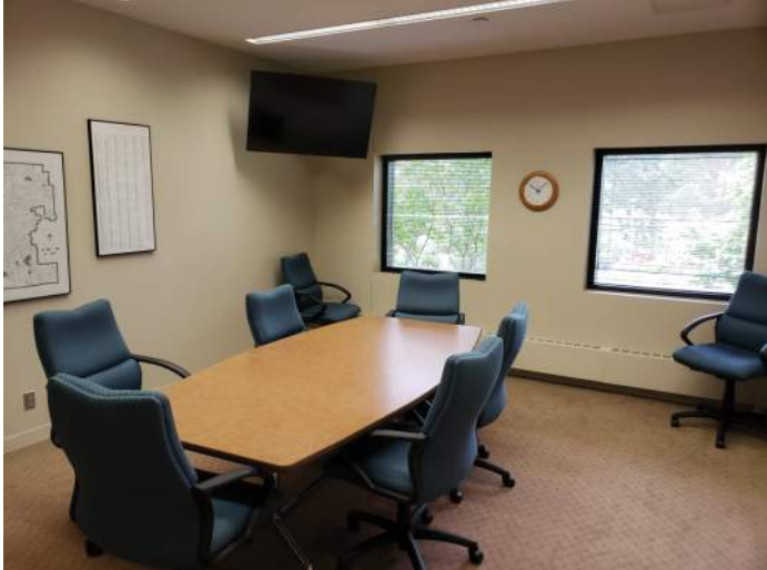
FIGURE 35: Carpet and ceiling tiles in Lake Rose Room are aged.
