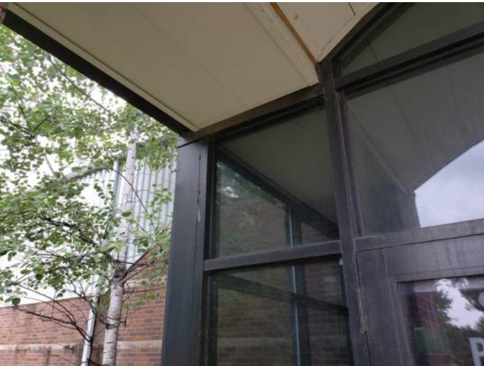
FIGURE 17: Paint finish on metal frame and door is failing and should be repainted.
