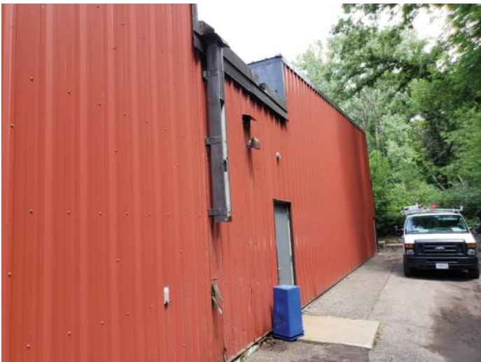
FIGURE 8: Downspout drains water onto wall and adjacent to building. Recommend extending downspout to direct water away from building.
