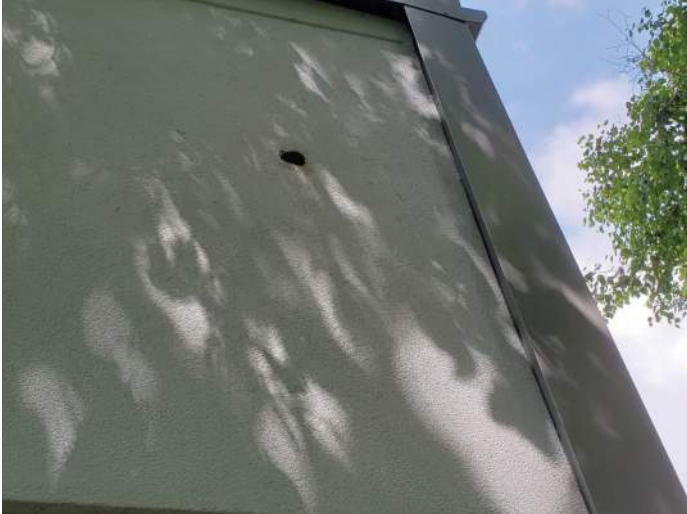
FIGURE 13: EIFS has multiple holes, likely from birds. Recommend repairing finish to prevent further deterioration of system.
