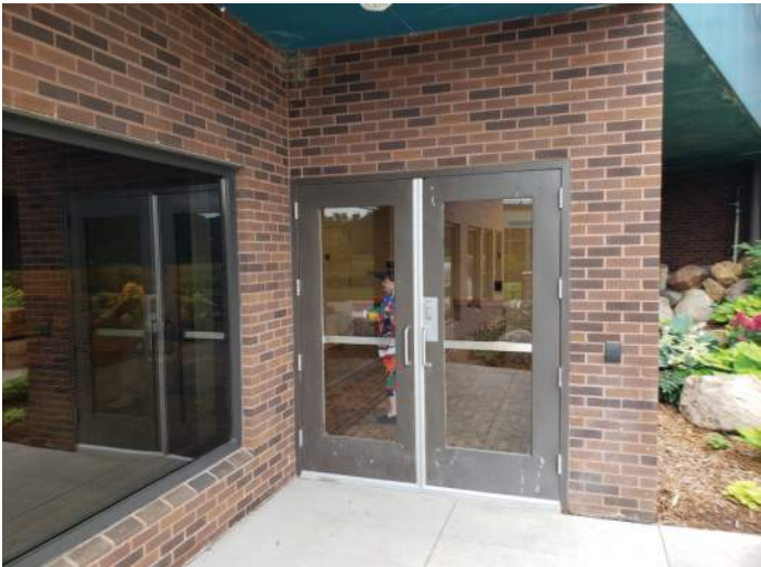
FIGURE 17: Paint finish on hollow metal door is failing and should be repainted.
