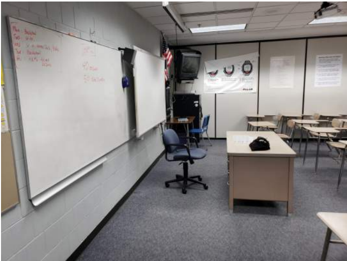
FIGURE 8: Classroom space, worn/stained carpet.
