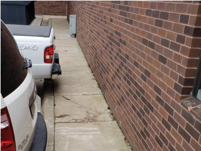
FIGURE 3: Concrete sidewalk is cracked and spalling near loading area.
