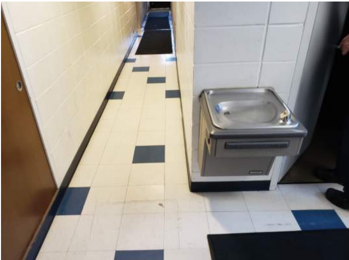
FIGURE 11: Worn floor finish in corridor/lobby.
