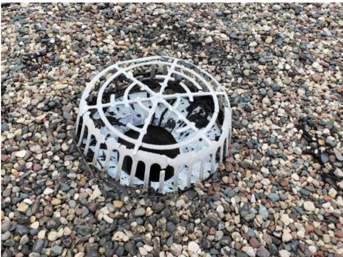
FIGURE 21: Roof drain screens are deteriorated and should be replaced.
