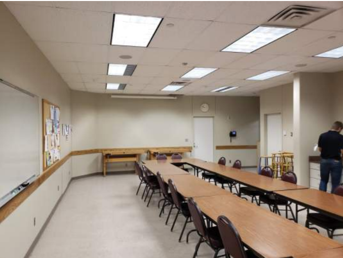
FIGURE 28: Floor and ceiling finishes in Minnetonka Mills Craft Room are worn.
