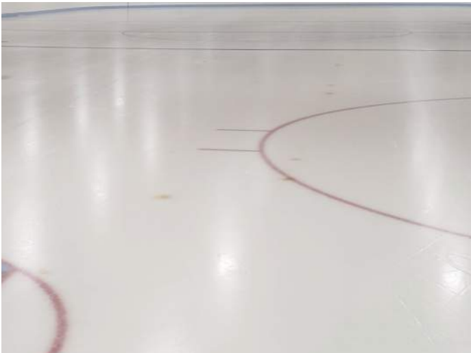
FIGURE 44: Brown stains on ice from condensation at ceiling. City is not sure if roof is leaking or if moisture is trapped in insulation panels.
