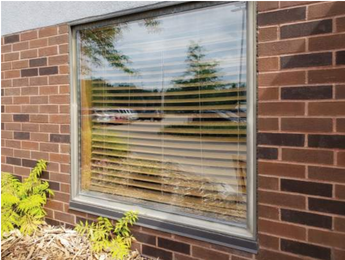
FIGURE 1: Windows are aged and past useful life expectancy. Replacement of windows is recommended.
