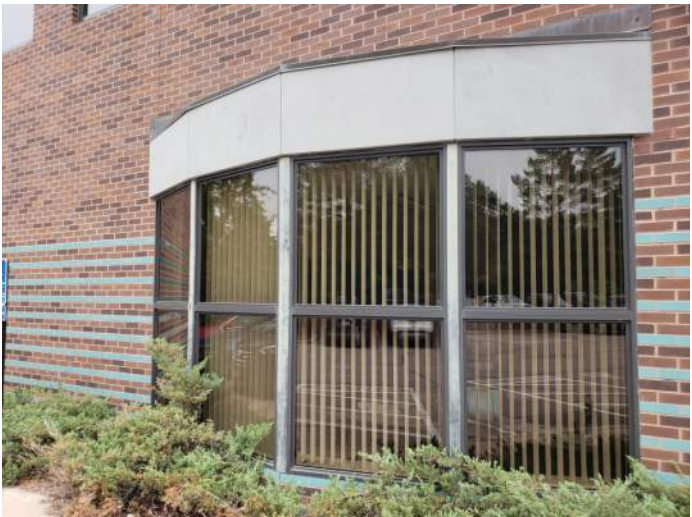
FIGURE 9: Metal panels are discolored and faded. Recommend repainting metal panels.
