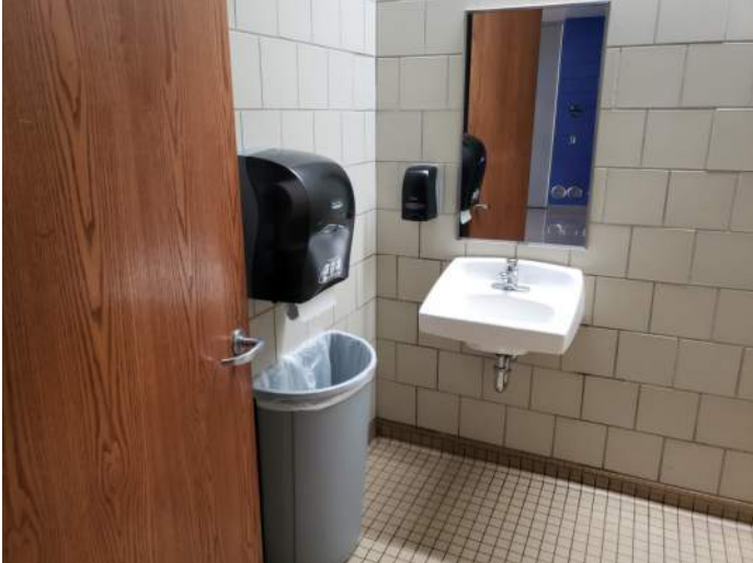
FIGURE 13: Lavatory missing pipe protection as required by ADA guidelines.
