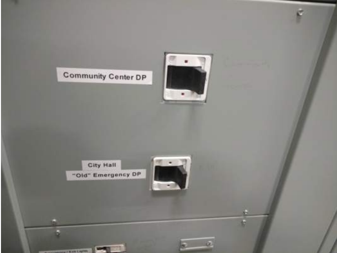
FIGURE 42: Disconnect for Community Center Distribution Panel on City Hall Switchboard
