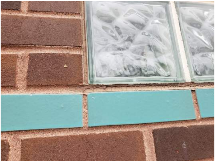
FIGURE 8: Sealants around glass block are dried and cracking. Sealants should be replaced to prevent water intrusion.
