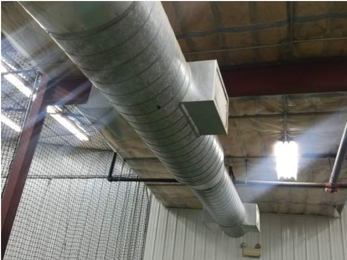
FIGURE 39: Batting cages only supplied in one location. Consider supplying evenly across area and integrating fans to destratify room.
