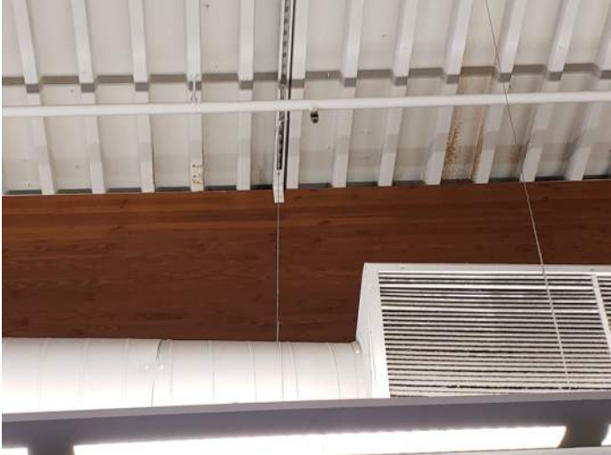
FIGURE 29: Rust is visible at underside of roof deck in fitness room.
