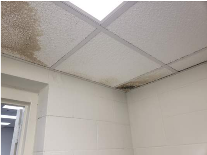
FIGURE 9: Stained ceiling tiles in corridor/lobby.
