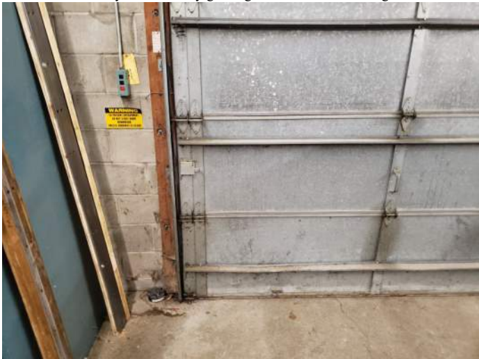
FIGURE 35: Overhead door at Arena B does not appear to have safety sensors installed. Recommend installing safety sensors at door.
