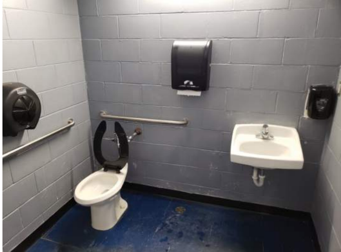
FIGURE 40: Restroom does not comply with MN Accessibility Code requirements. Finishes are worn.
