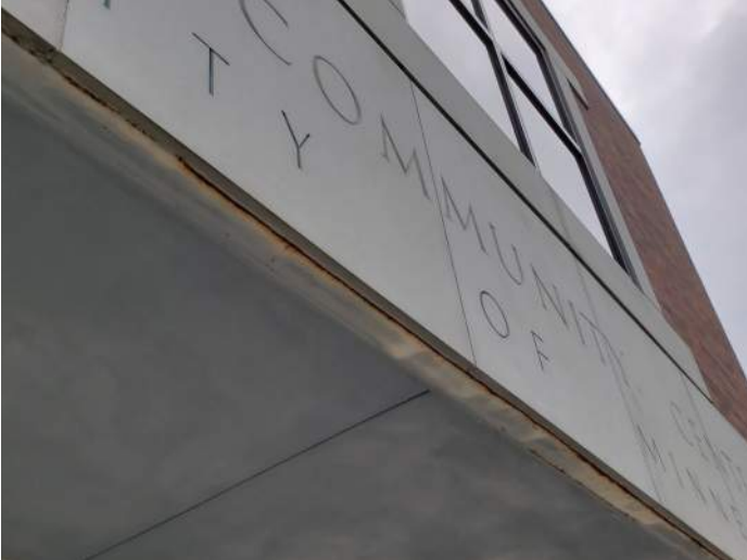
FIGURE 10: Rust is visible at underside of entry canopy. Recommend repainting and installing drip flashing to direct water from wicking into canopy.
