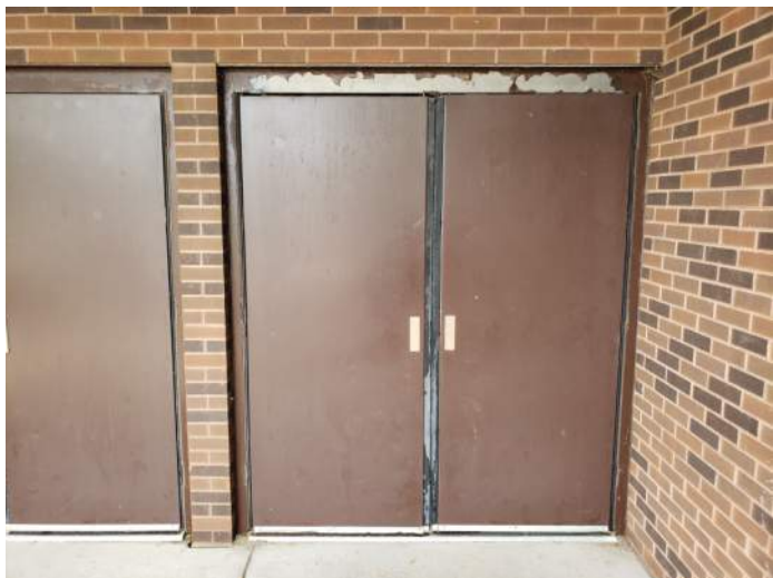
FIGURE 6: Paint at hollow metal frame is peeling. Recommend repainting the frames.
