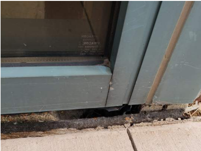
FIGURE 15: CMU block has deteriorated/chipped and a hole is present at base of wall. Hole should be filled and sealants replaced.
