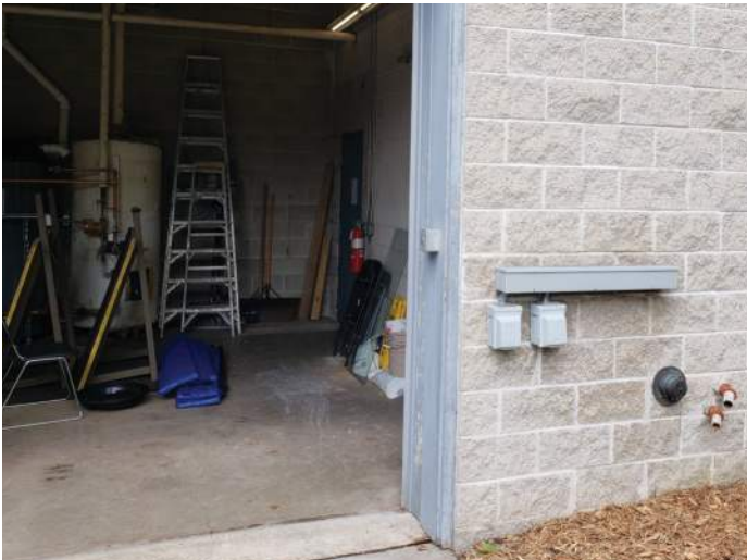
FIGURE 21: Overhead door jamb paint finish is peeling. Recommend repainting to prolong lifespan.
