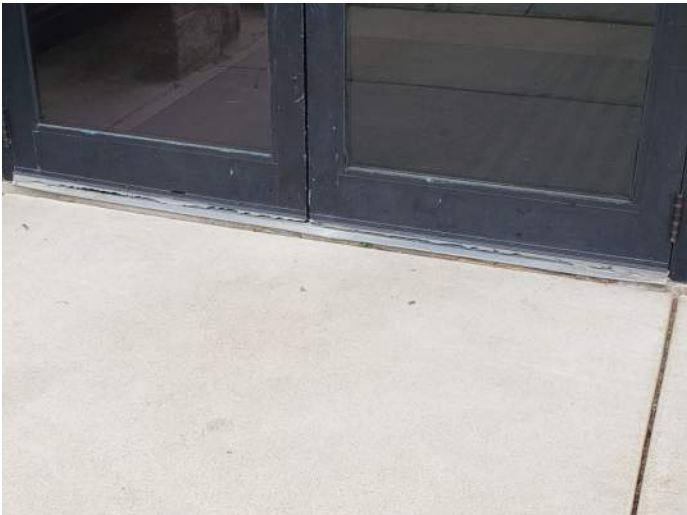
FIGURE 20: Weather seals at door threshold is torn and missing. Recommend replacement.
