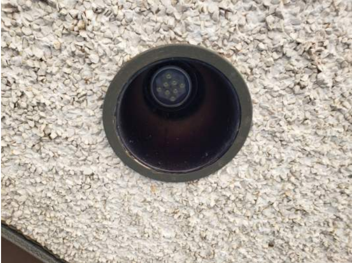
FIGURE 19: Exterior light fixtures retrofitted with LED lamps.
