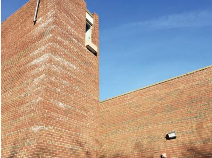
FIGURE 1: Efflorescence visible around the hose tower.
