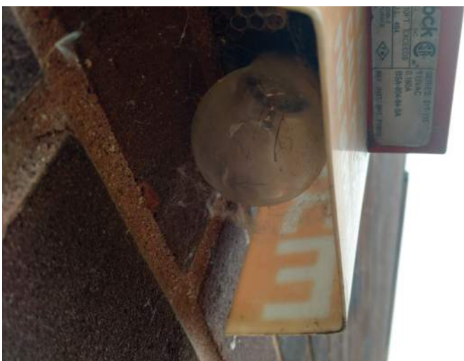
FIGURE 45: Incandescent bulb for dated fire alarm audio/visual device.
