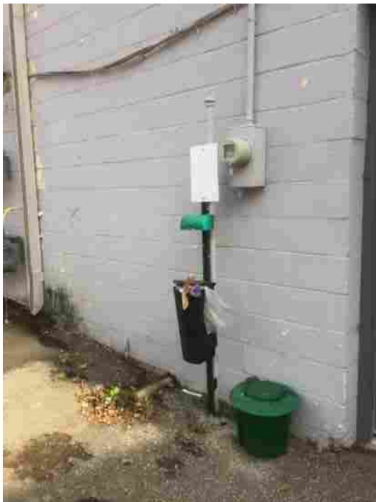
Photo 7: Horizontal pipe and vertical vent pipe possibly associated with the former septic system.
