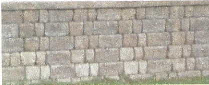
STACKED BLOCK RETAINING WALL LESS THAN 24" TALL.
