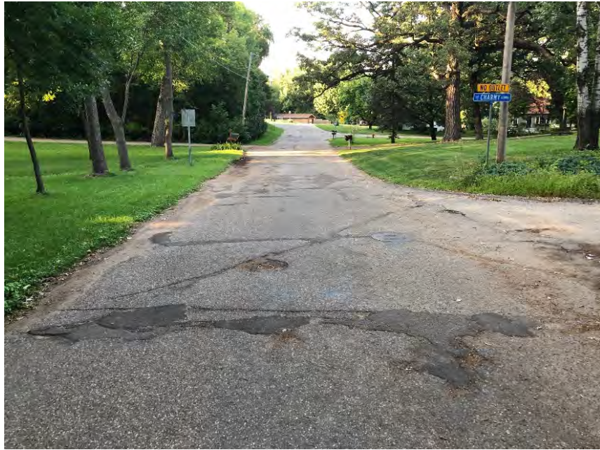
Photo 1 Existing Typical Pavement Condition – Groveland School Road Facing North
