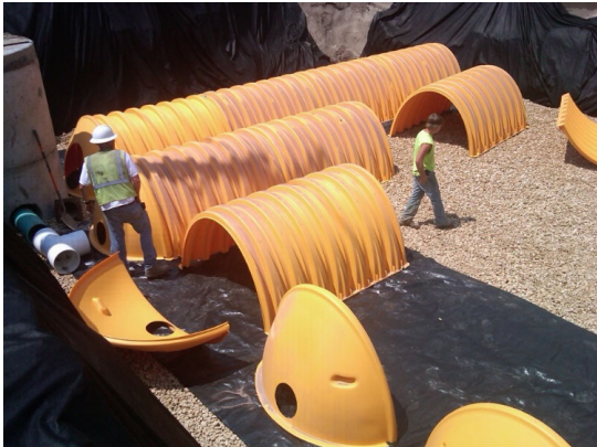
Underground Infiltration Chamber
